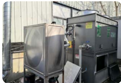
Cooling circulation tower
