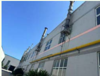
Combustion exhaust gas purification equipment
