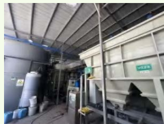
Wastewater treatment station
